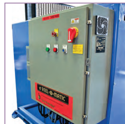
UL-508 Panel Box
